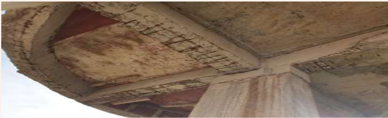
Figure 1. Typical Distresses observed in a newly built building in Delhi-NCR. [1]
